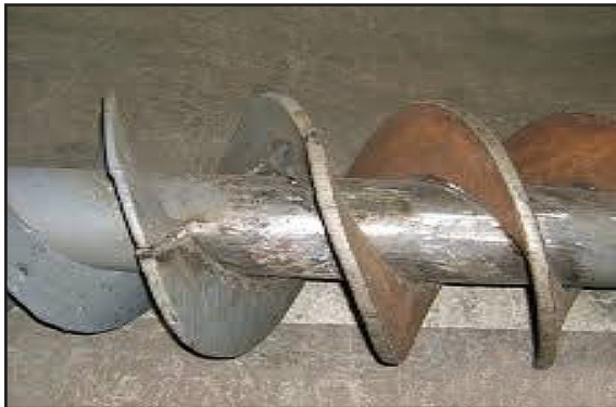
Screw is worn, cracking, and no longer efficient.
